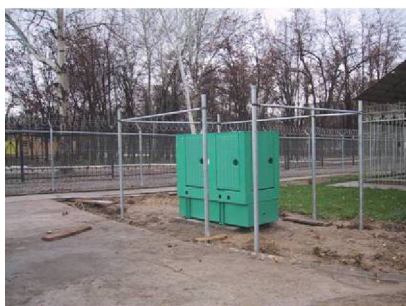
New Emergency Diesel
