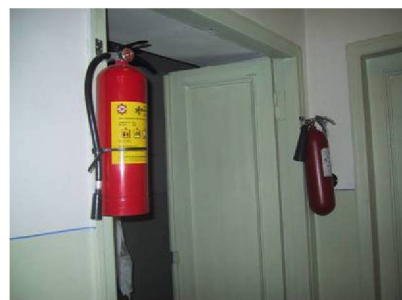
New Fire Extinguishers
